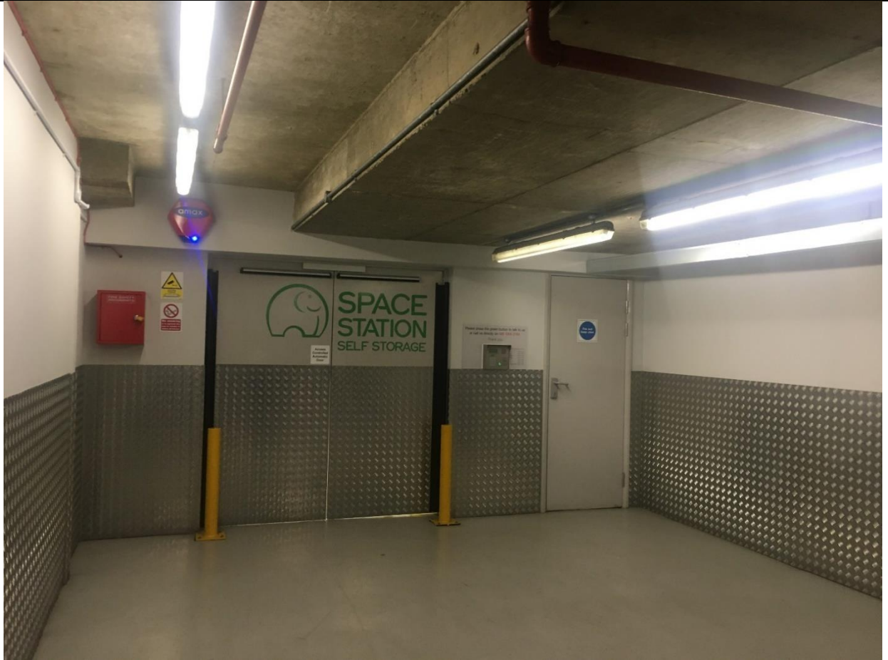
Existing self-service unit entrance and loading area at level 1 within the car park
